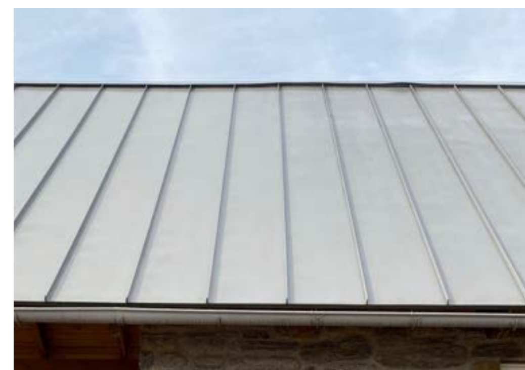
EXTERIOR FINISH - STANDING METAL SEAM
