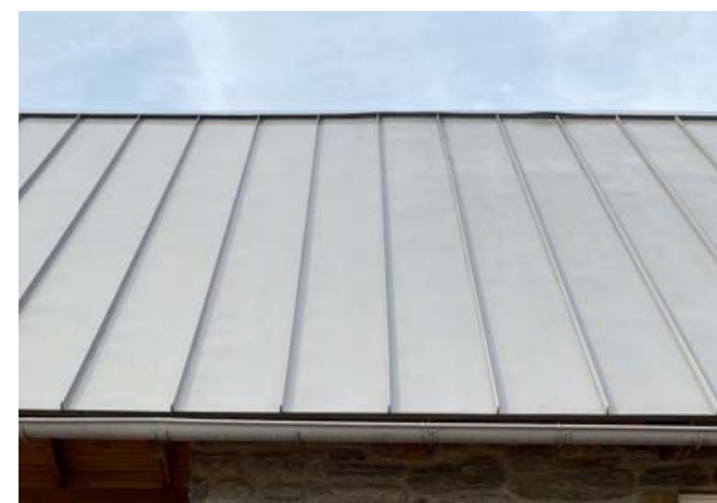
EXTERIOR FINISH - STANDING METAL SEAM
